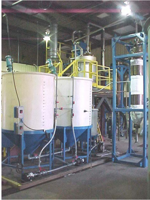
Figure 1: Waste Feed Surrogate Preparation Batch Tanks
